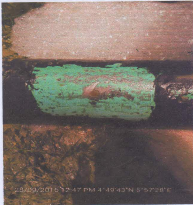
Fig 3: Leak point (drilled hole)
